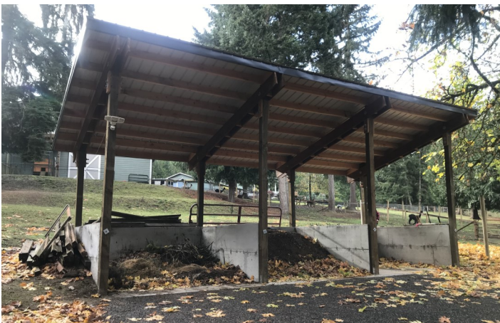
A completed waste storage facility designed and built to assist with the safe storage and composting of manure. Capturing and covering of the manure decreases excess nutrient runoff.
